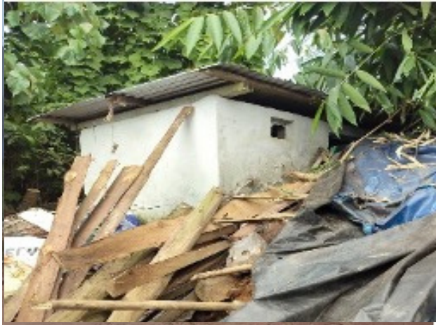
Flood-damaged house in Mirik
