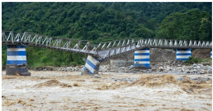
Damaged Dudhia Bridge near Mirik
