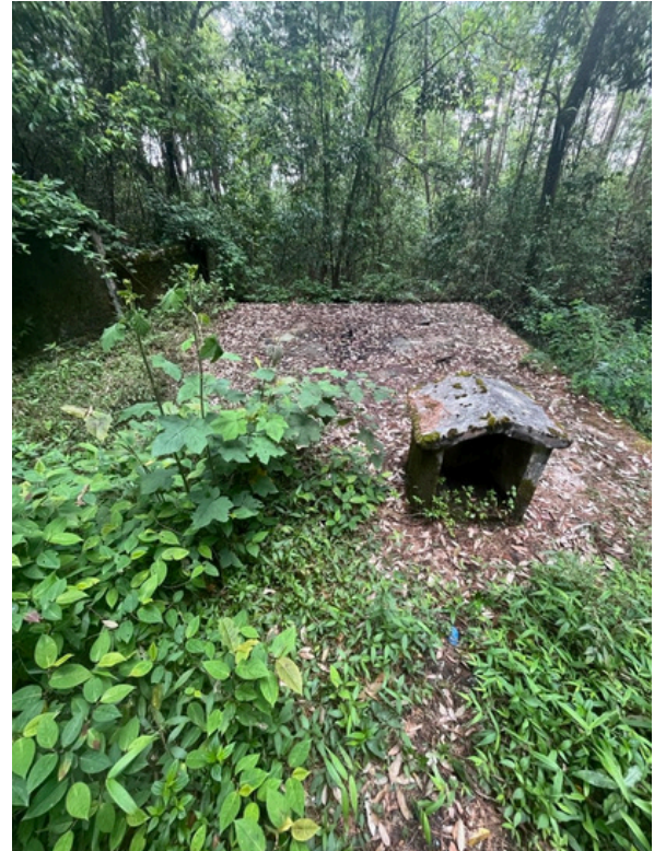
Photo 2: Water Collection Reserve
